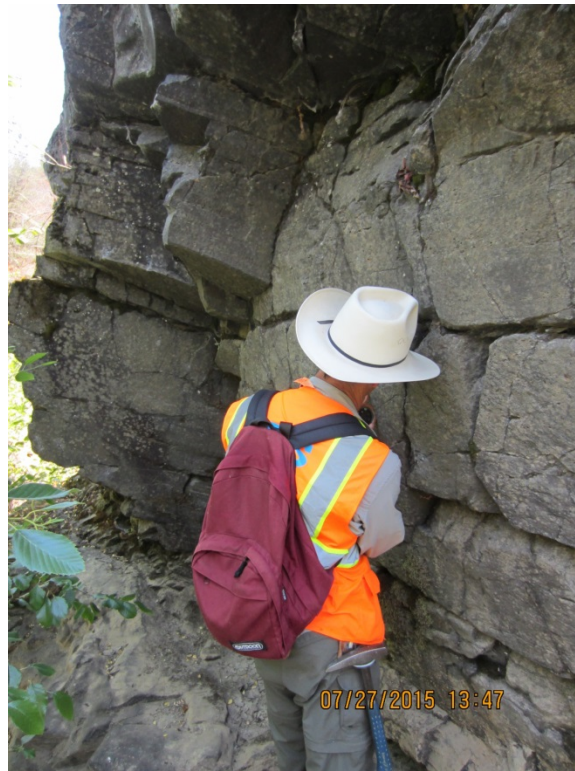
Photograph 5. East facing view of typical discontinuities in outcropping bedrock (massive basalt) at the toe of slope along the south bank of Bear River
